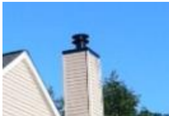
Chimney Metal/Rim Cap and Vent on home that originally had/has a wood burning fireplace.
